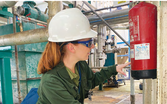
Conducting routine check on expiry dates of fire extinguishers at BOH, Spain
